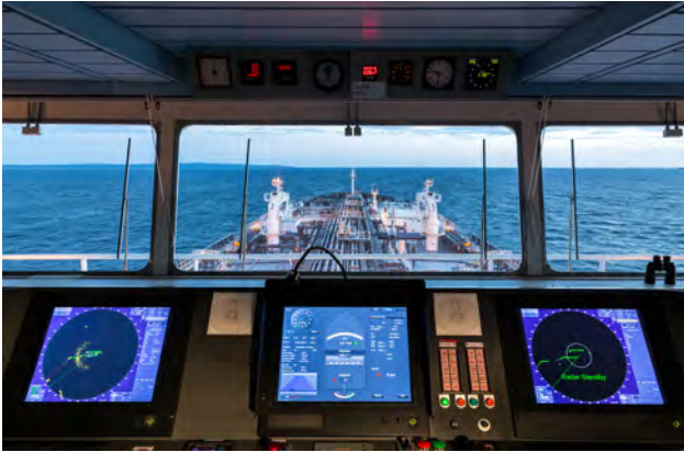
Figure 1: The NMEA 2000 application profile for maritime electronics is especially used in navigation systems (Source: Adobe Stock)
